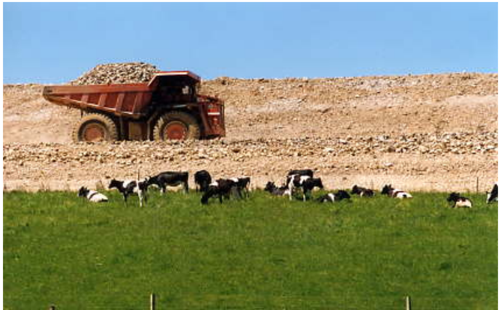
Stock on Rehabilitation Areas of Waihi Gold's Waste Rock Embankment Courtesy of Newmont Waihi Gold
